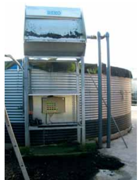
Thanks to container cultivation and water recycling there is a closed system. Germs are eliminated by means of a sand filter.
