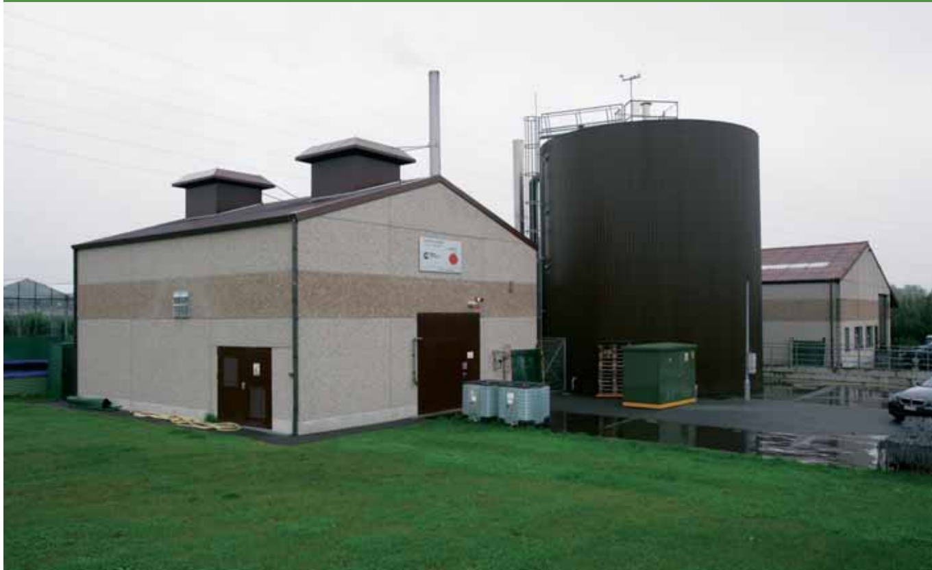
If all challenges are met at the same time, a combined heat and power system is cost-effective.
